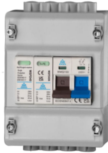
Single phase meter Isolation c/w surge protection
